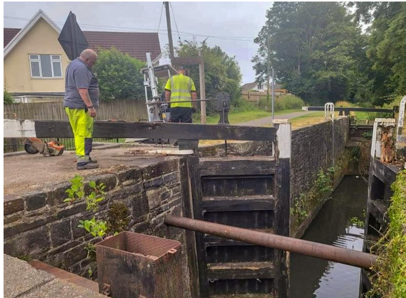
The old gates being removed on lock 21 adjacent to the Fourteen Locks Canal Centre
