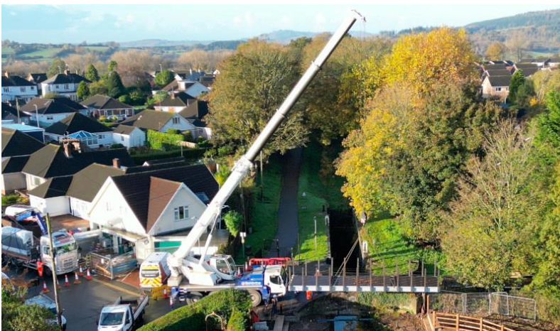
The new footbridge being lifted into place adjacent to the Fourteen Locks Canal Centre. Photo by "Court Above the Cut".
